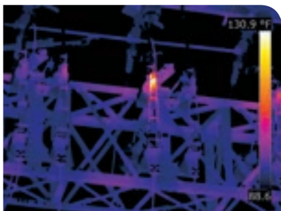
Overheating substation circuit breaker
