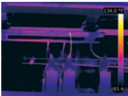
Hot power line transformer
